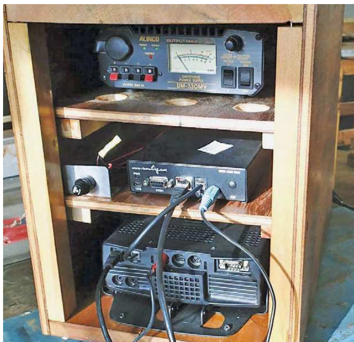
The front of the remote station in a box as it was being wired. Note the small fuse block to power the RRC box. From top to bottom: the 12 V power supply, RRC radio unit, and TS-480SAT transceiver in a mobile mount bracket. The top interior shelf shows the holes for flow-through cooling.
