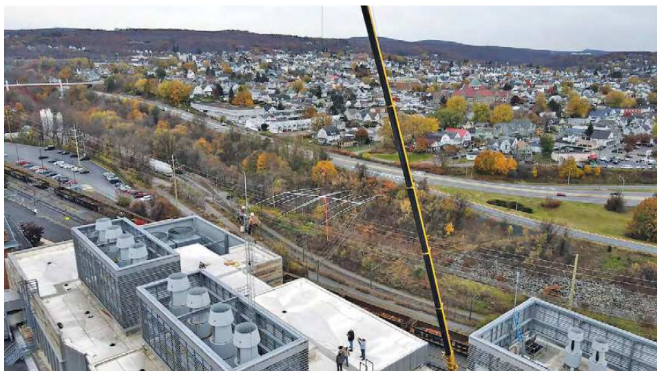
A crane lifts an antenna into place for W3USR's new location. [Byron Maldonado photo]
