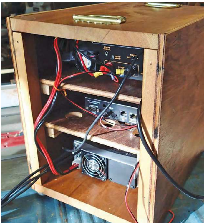
The back of the station in a box as it was being wired.
