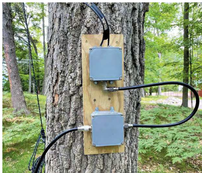
Figure 5 — The balun, toroidal transformer, and coaxial/ferrite common-mode current choke were placed in two 4 × 4-inch waterproof plastic electrical boxes and mounted to a tree.
