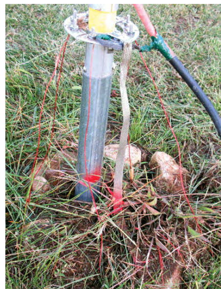
Figure 2 — The lower radial wire plate, along with the coaxial connections and ground rod cable. [Robert W. Lobenstein, WA2AXZ/9, photo]
