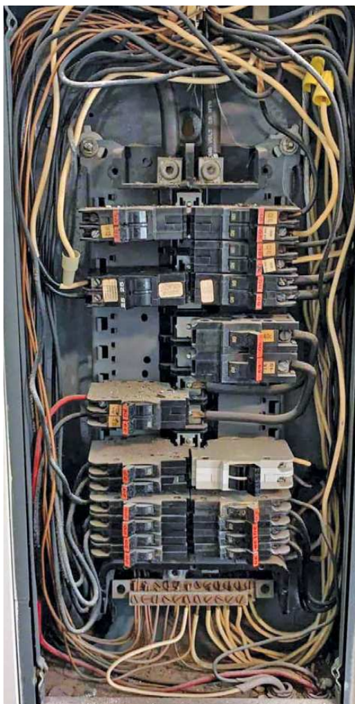
Figure 1 — An example of a split bus panel. These panels contain two separate sets of bus bars. [www.waypointinspection.com]
