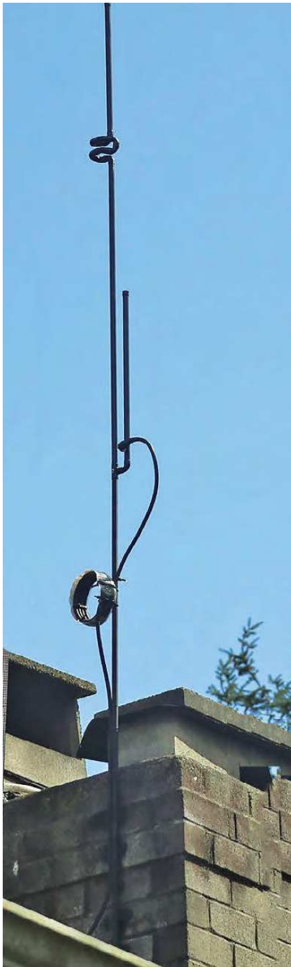
Figure 4 — The roof-mounted saxophone antenna. The coiled choke balun shown is a poor choice. A much better solution would be two to three turns of the coax through a mix-31 toroid.
